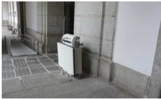
Platform lift in Patio del Abrevadero.
